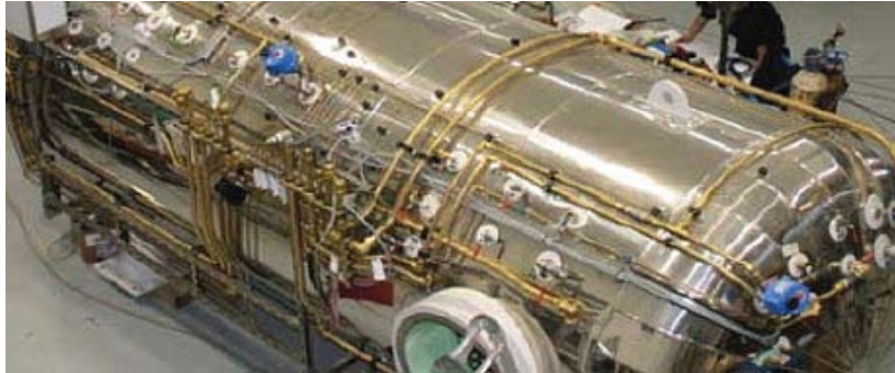
Tungum tubing installed on a saturation diving system module
